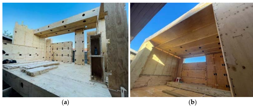
Figure 3. Skylark 250 assemblies with modifications. In (a), there is progress up to the beginning of the ceiling installation, and in (b), there is only one missing facade.
